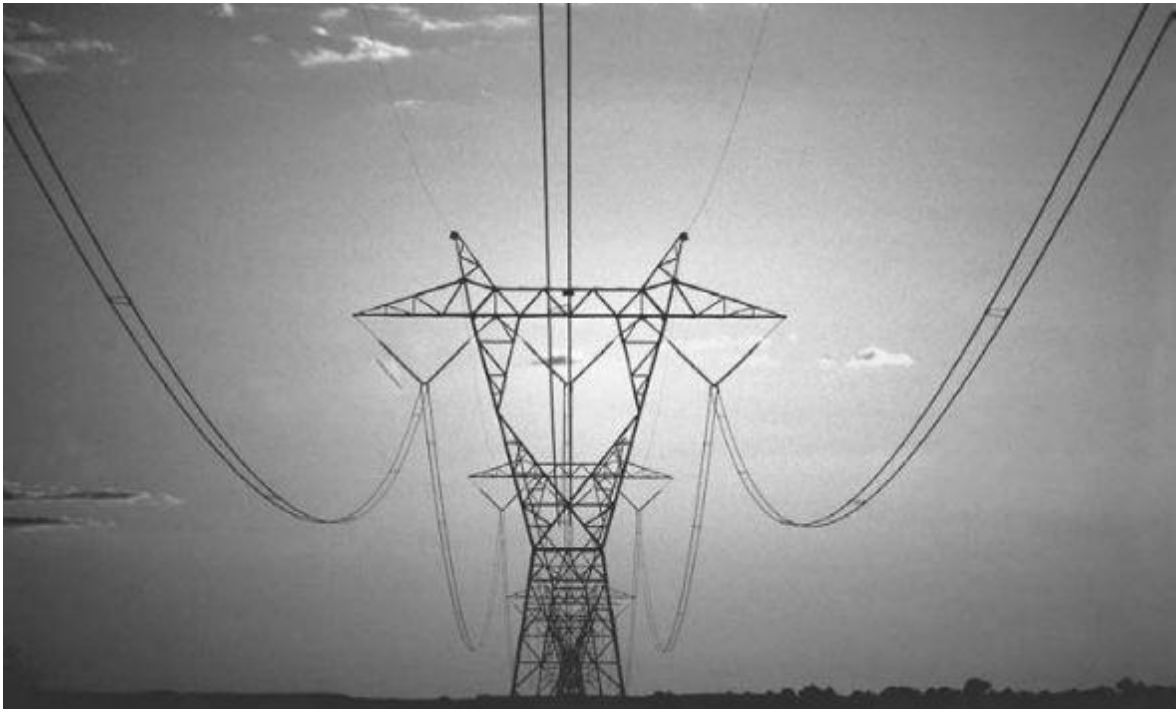
Figure 40: High-voltage transmission lines [54]
